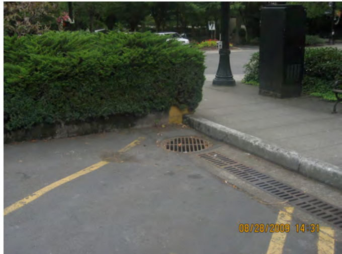
Photo 8. Direct storm drain connection to Streams Typical parking lot drain
