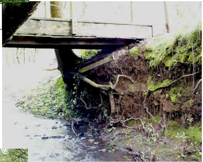
Photo 2. Severe stream bank erosion Springbrook Creek
