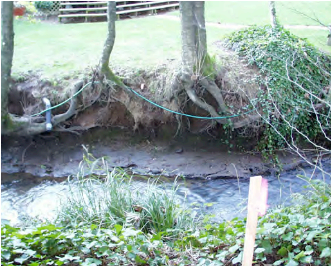
Photo 10. Property damage & safety hazard Springbrook Creek
