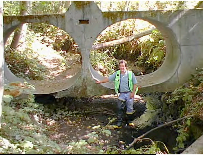
Photo 4. Channel incision Springbrook Creek
